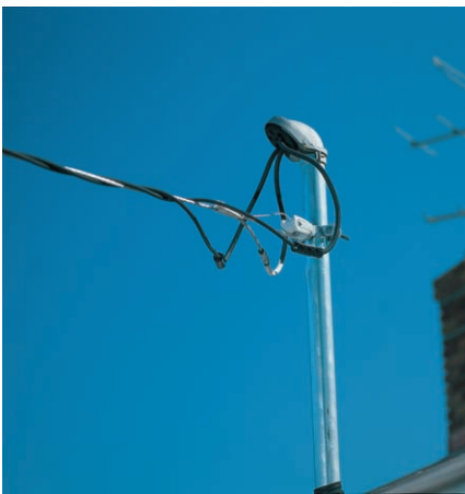
Electrical service mast.
