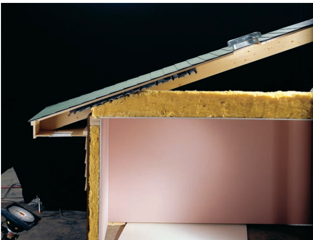
Unfaced batting between attic joists must leave room for proper attic ventilation.
