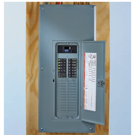
A main breaker box. The empty spaces under the breakers are potential new circuits.
